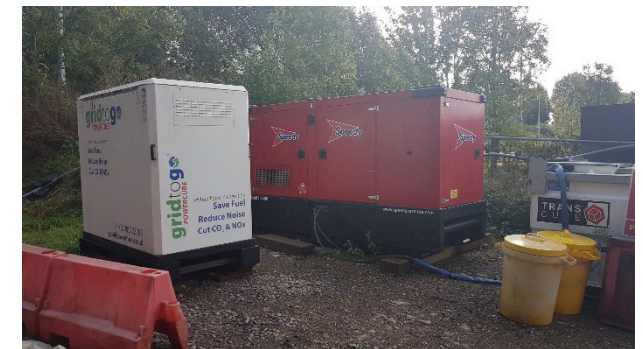
Figure 3 – Generator and Battery Bank
